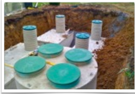
2,000 gpd decentralized on-lot MBR plant for a grocery store and a restaurant in Pennsylvania
