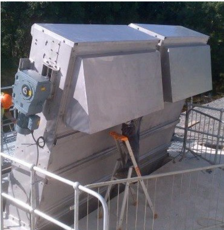
Discharge chutes from dual CBS screens
