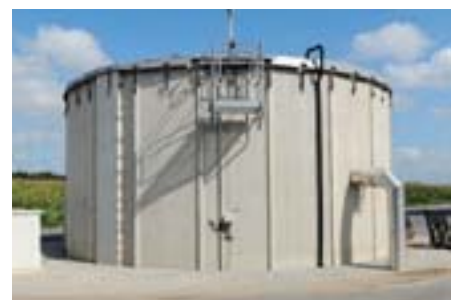
This container is used as an intermediate storage for manure
