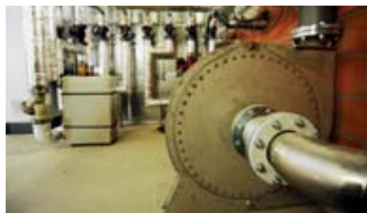
The compressor increases the gas pressure to 90 mbar, so the biogas can later be used in the CHP.
